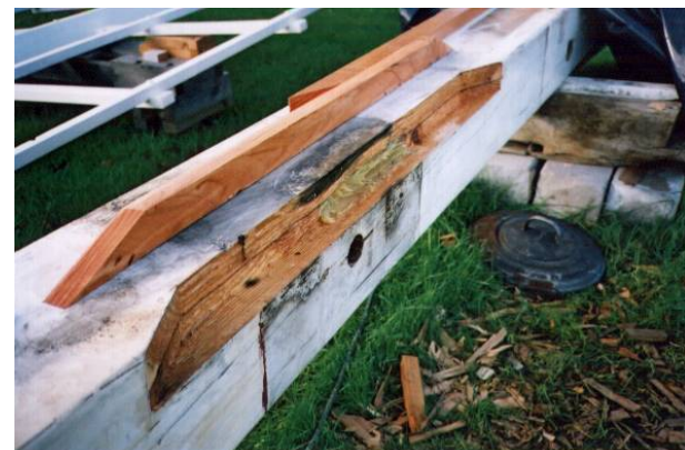
Splicing in new material at the middle of the stock, using epoxy resin adhesive and dry preservative plugs embedded in the old timber
