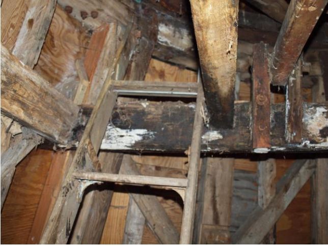
Fig.9 Fungal attack 2. Other side of hursting beam, and curb
