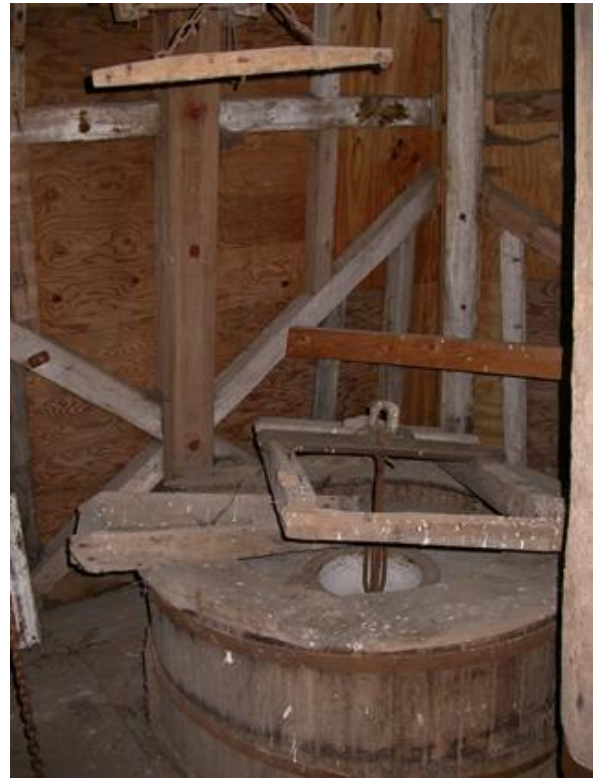
Fig.3 Strengthening and re-cladding the smock (G.C. Wilson holding operation): additional framing, and plywood cladding.
