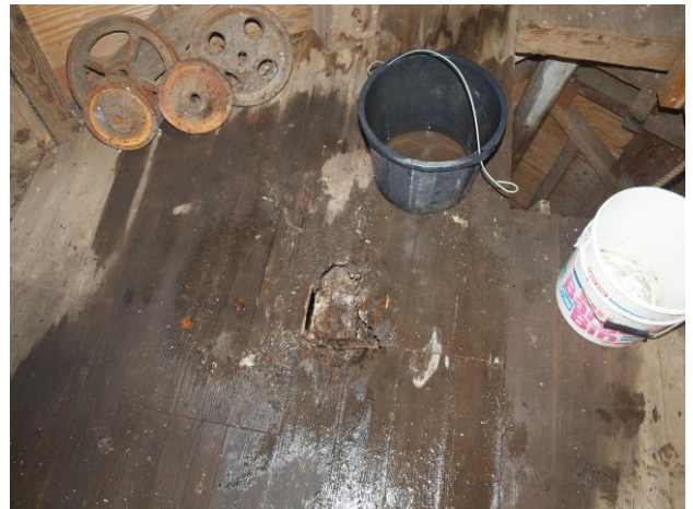
Fig.12 Damage to Bin Floor, from continual wetting
