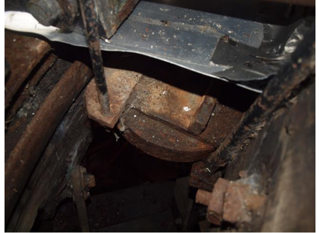
Fig.11 Holding Operation aluminium guttering, instasly to channel rain water out of cap and over top of Curb
