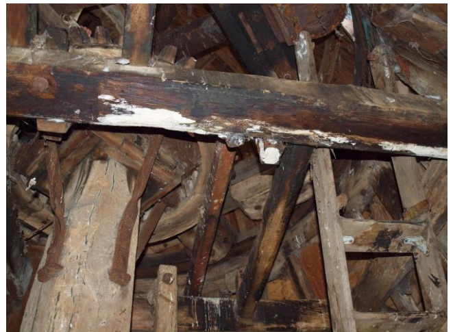
Fig.8 Beginnings of fungal attack on beams of hursting near tower top, caused by many years of damp ingress
