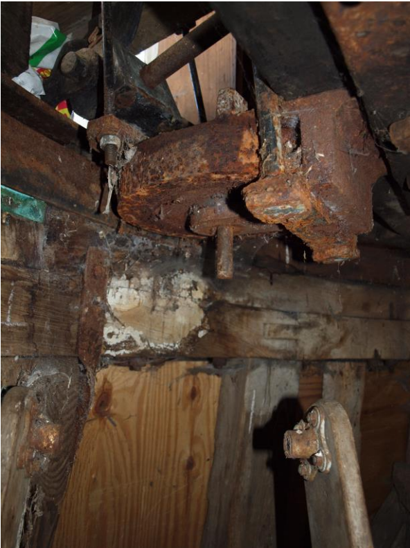
Fig.10 Curb, and pronounced rusting of rear cap Centring Wheel
