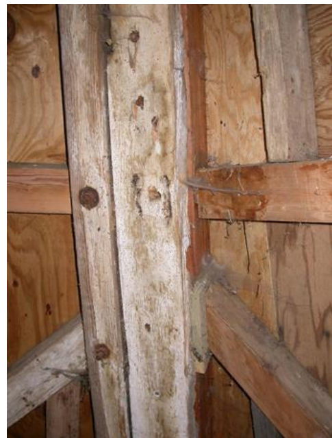
Fig.4 Strengthening & Re-cladding the Tower (G.C. Wilson holding operation): plating a cant post and cladding with plywood sheets
