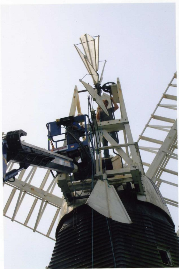
Fig. 13 Lowering a fan blade for storage (R. Bramley in 'cherry picker, A. Kite on cap)
